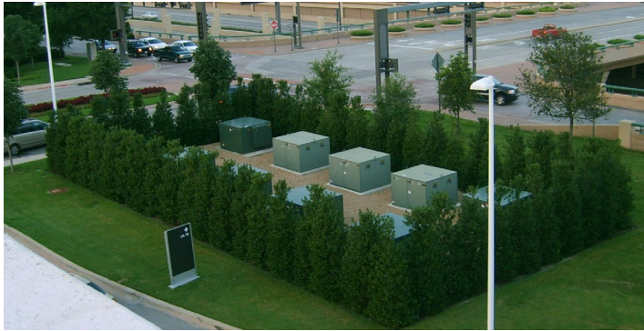
Figure 4.07.6. Example of Screened Ground-Mounted Utility Equipment
